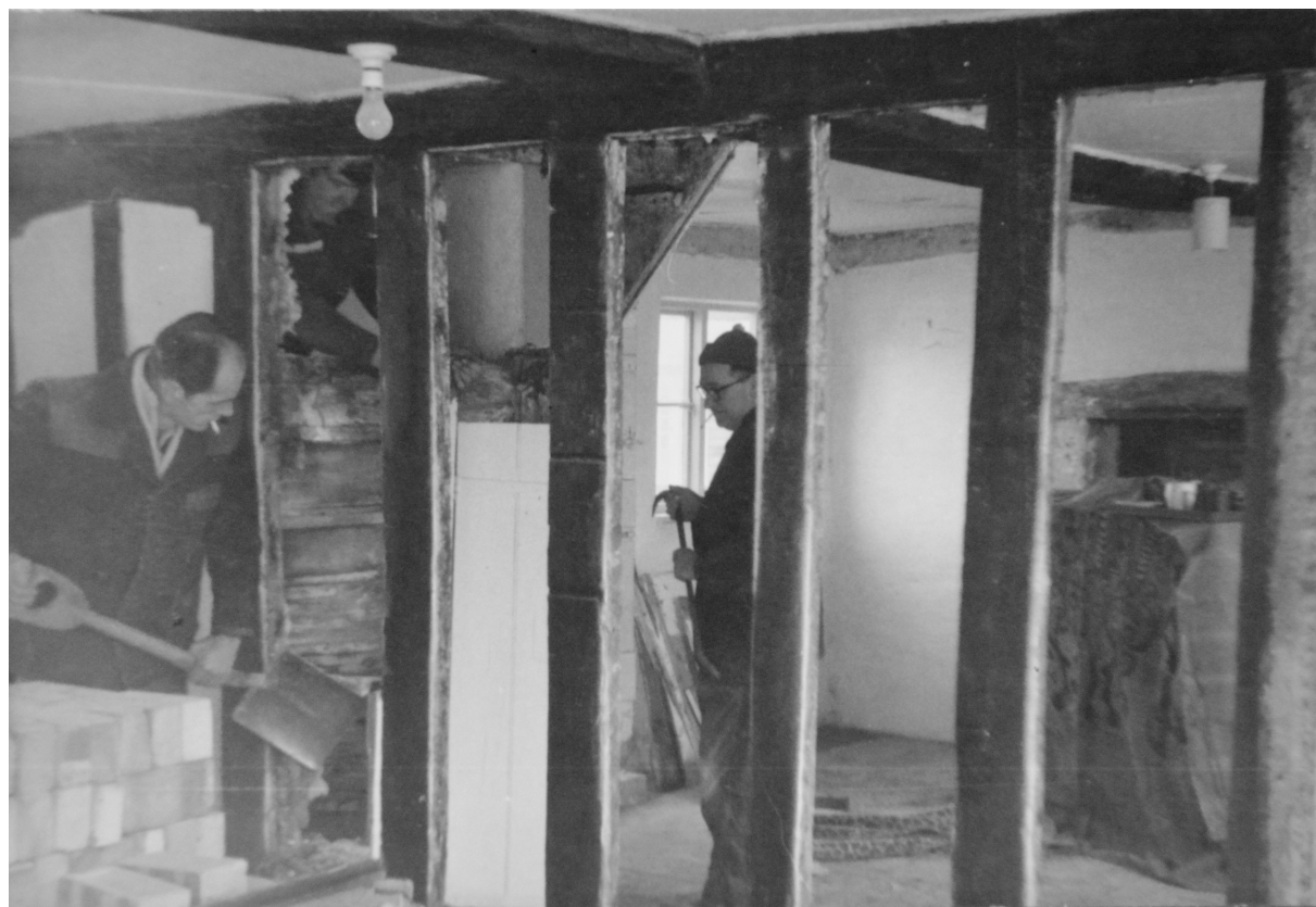
Photo 8. Clearing rubble in No. 46 High Street, that revealed hidden door on left with arched top.
